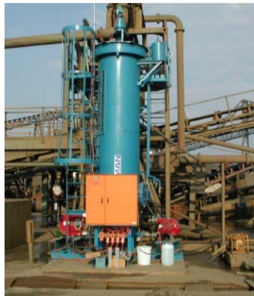
Figure 5: Paste Thickener Pilot Plant
